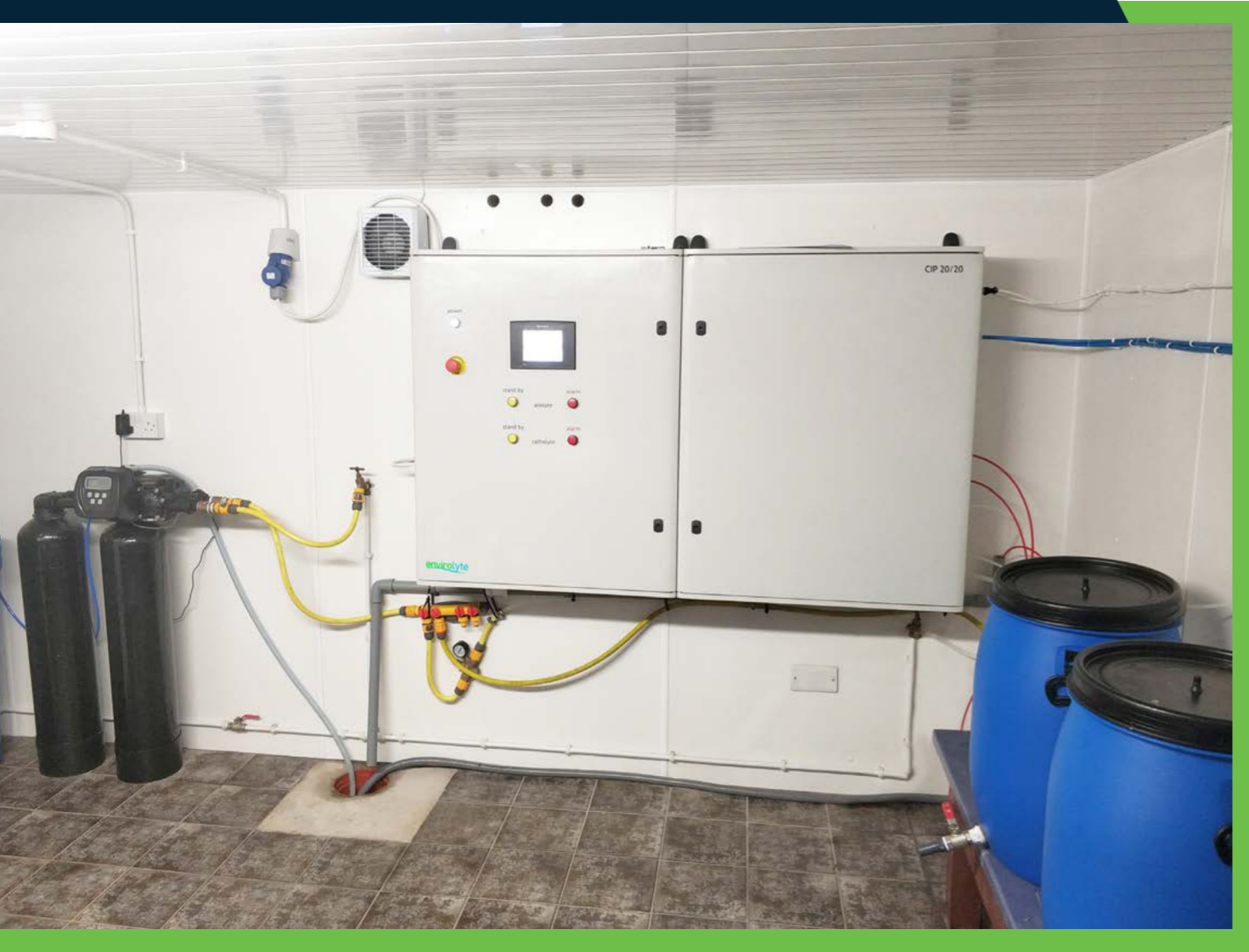
Photo installation courtesy of Envirolyte
