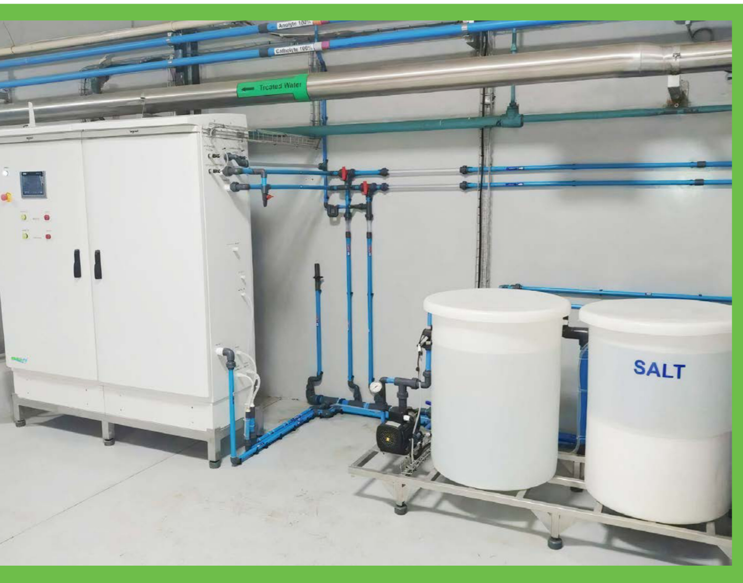
Photo installation courtesy of Enviolyte
