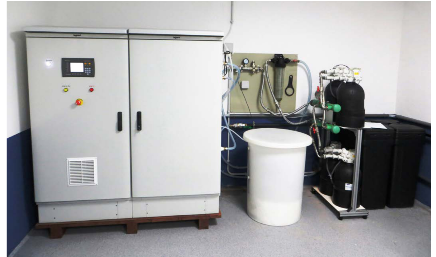
ELA 18000 generator installation and accessories
